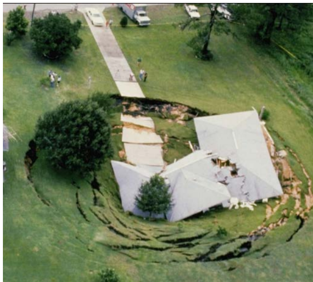
Figure 3-19 Home Swallowed by Land Subsidence
