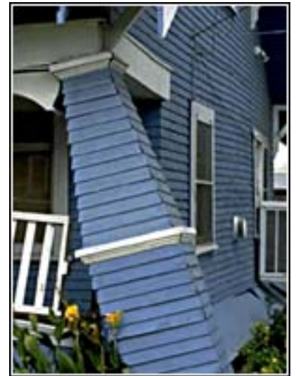
Figure 3-6 Earthquake Damaged Porch
